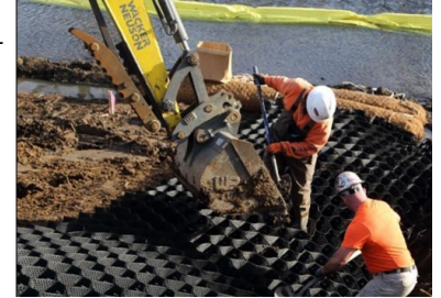
At Constitution Park, the riverbank was reinforced using 12-inch-high, honeycomb-shaped grids filled with sand and biochar.
