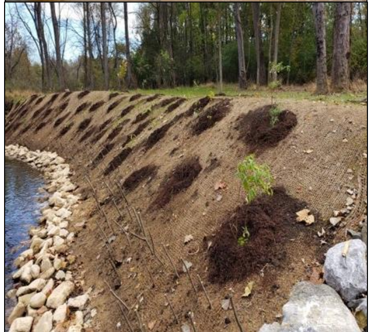
Native trees and shrubs were planted on the riverbank to enhance the habitat and provide stabilization.
