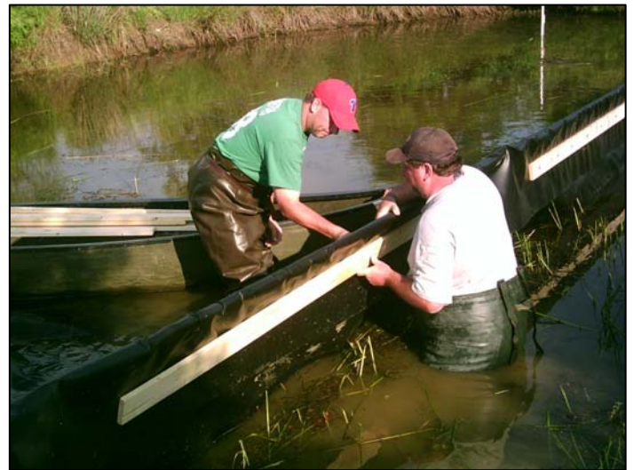
After installing the posts and rail, the Science Team installed a liner to make sure that water would not pass through the barrier. Sandbags were placed on the bottom of the pond on top of the liner.
