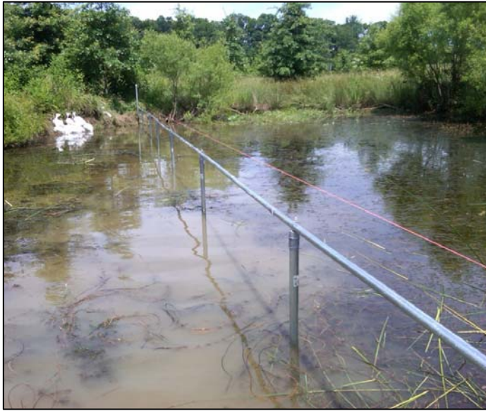
To create the barrier, the Science Team installed posts into the bottom of the pond and then placed a top rail across the posts.
