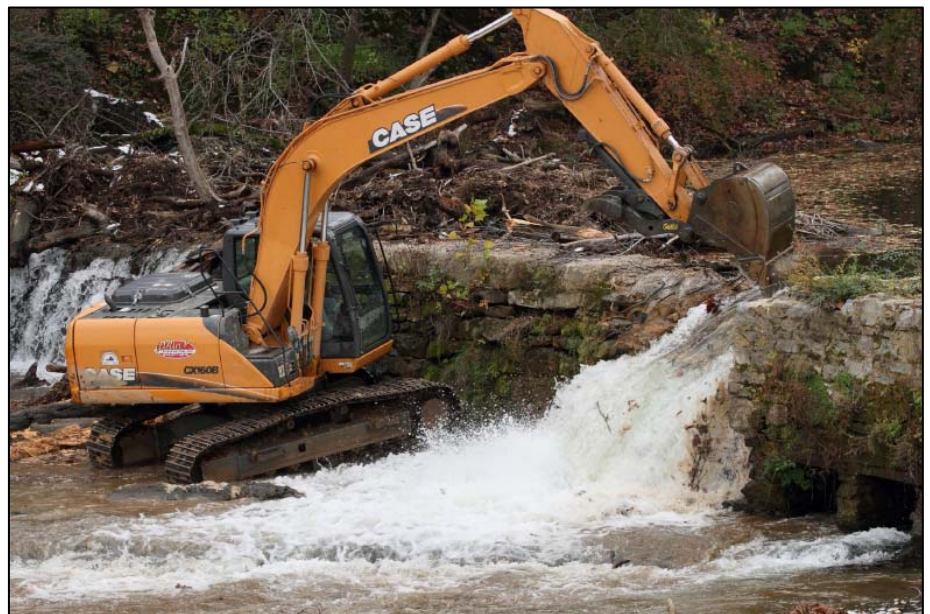
An excavator begins the process of removing Rife-Loth Dam on October 31, 2011. (Photo courtesy Mark Miller – www.markmillerphotography.com ).
